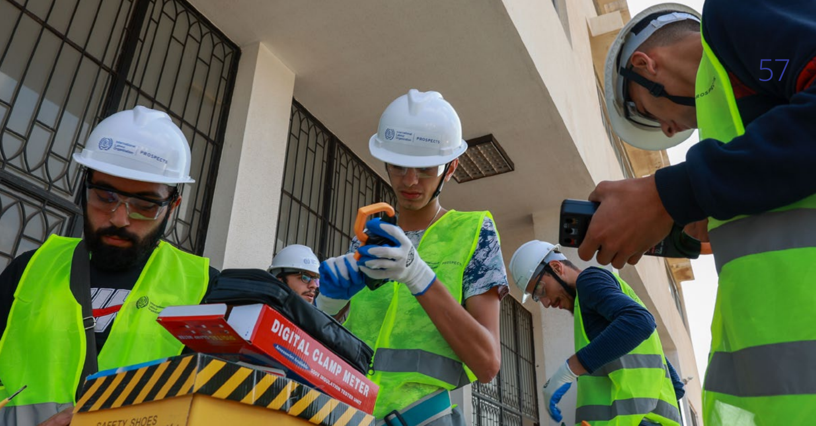
Students wear OSH gear and equipment before installing solar panels on the roof of one of the TVET schools in northern Lebanon.
