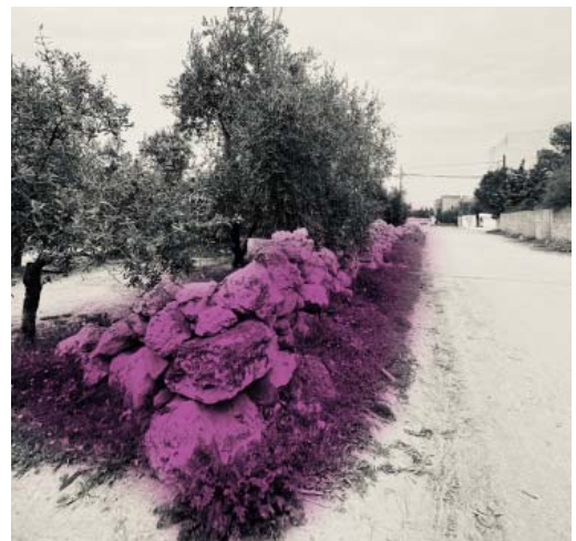
Dangerous Stone Fences
