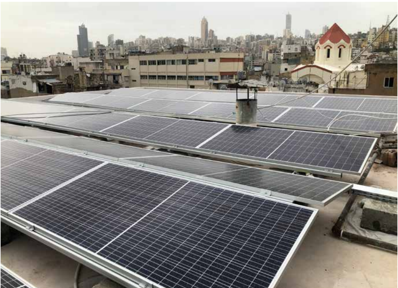
Solar panels installed on the roof of the community centre in Maraach, Bourj Hammoud
